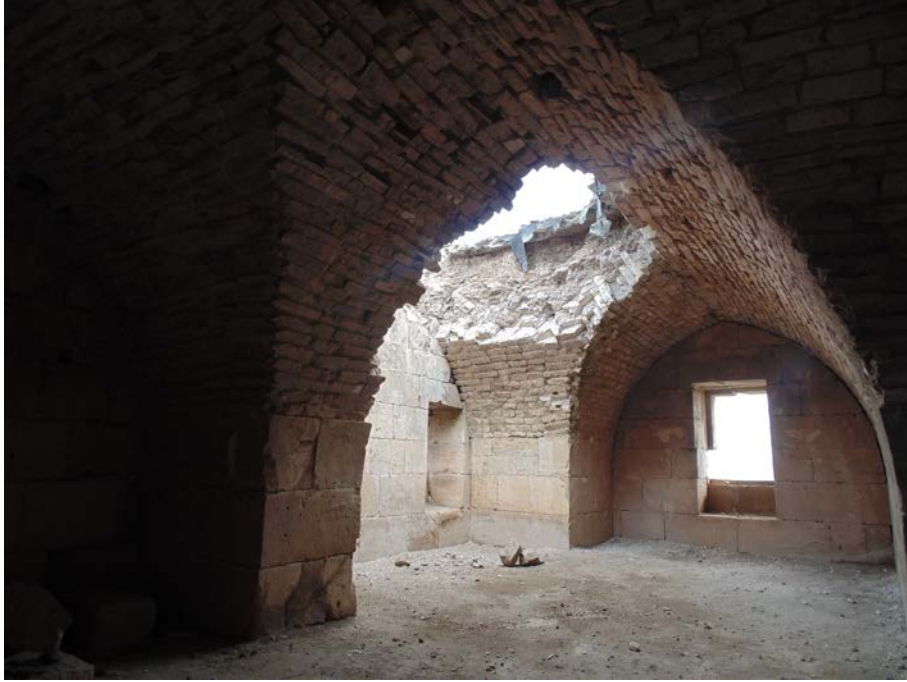
Leader Tower in Krac des chevaliers(After) - © DGAM 2014
