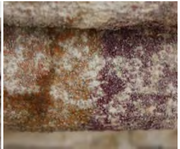
Fig. Biological damage
