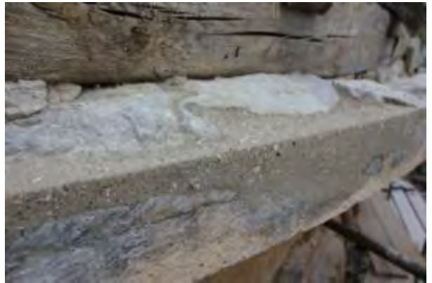
Fig. After the reconstruction
